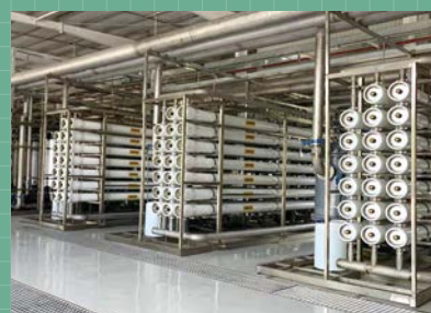
Reverse osmosis (RO) water treatment system for reusing water
